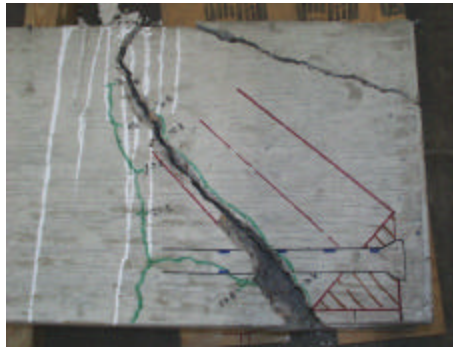
i. Side View - Exterior Cracking
